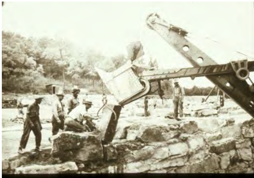
Crane at Twin Lakes, setting stones in place for the spillway, ANF
