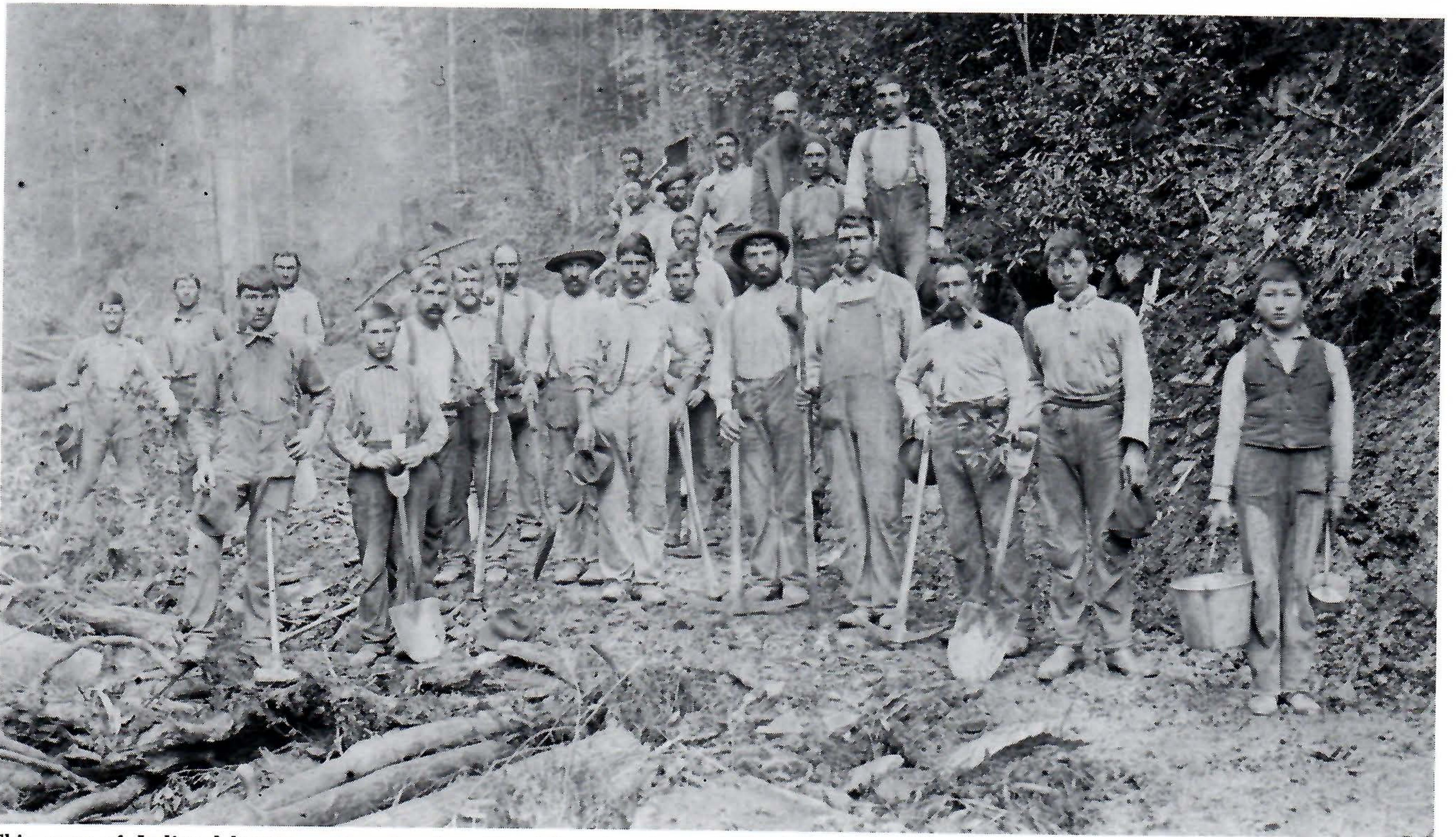
This crew of Italian laborers, equipped only with picks, shovels, and wheel barrows, will dig the right of way along the hillside for a new spur line of the C. & B. F. Note the waterboy at the right — a most important member of the crew.
